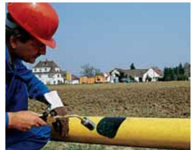
PERP application on factory coated PE pipe Heat-applied repair patches with their excellent adhesion to commercial, factory-applied coatings provide a virtually monolithic coating repair of high quality.
